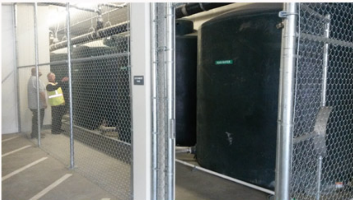
After their installation Bobby trained building maintenance how to operate the tanks.
